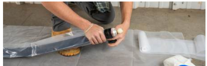
PERFORM A TEST RUN TO ENSURE THAT THE PACKER CAN REACH THE POINT OF REPAIR WITHOUT ISSUE.
